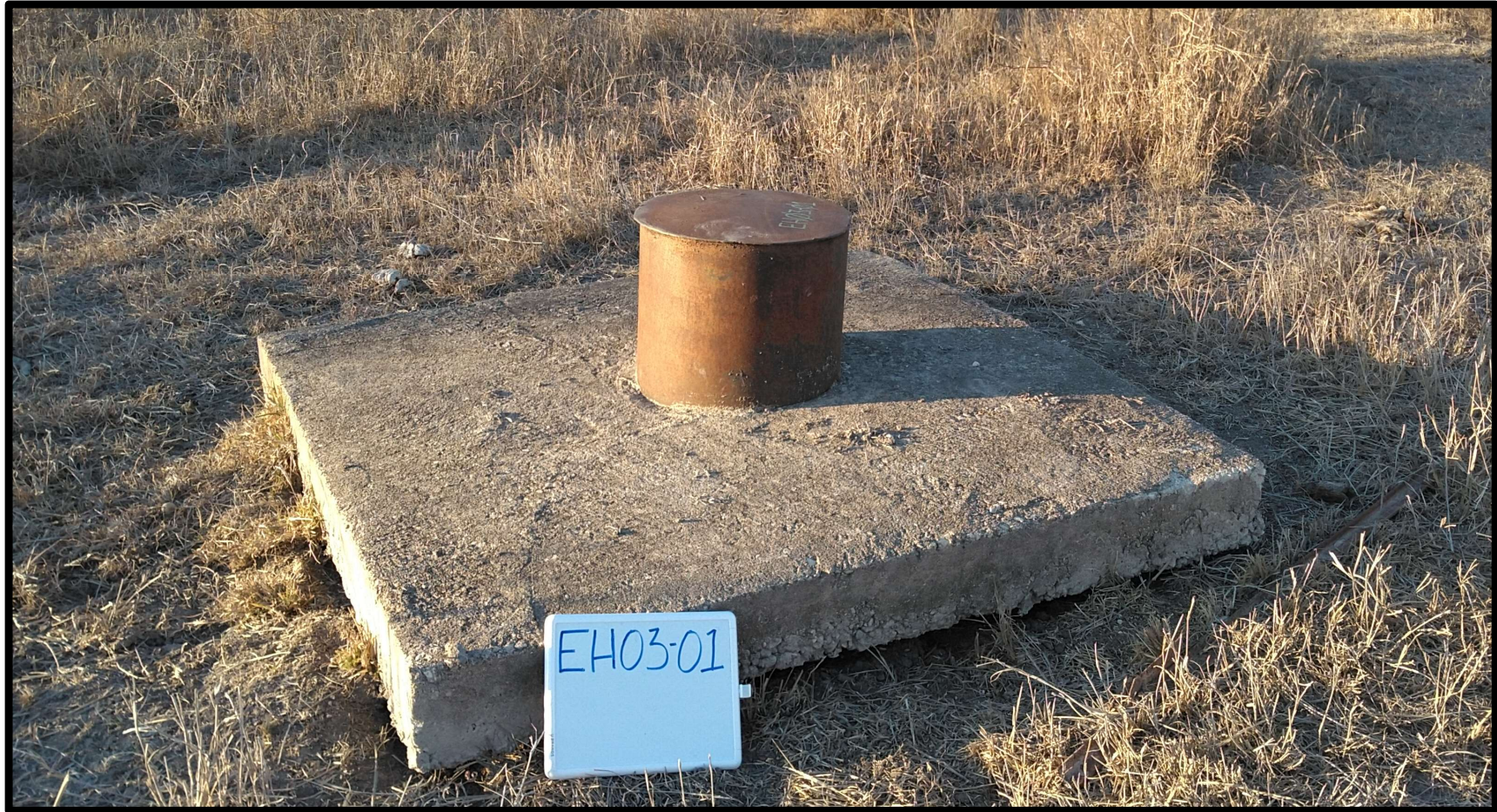
Non-operational Permitted Well – No Meter
