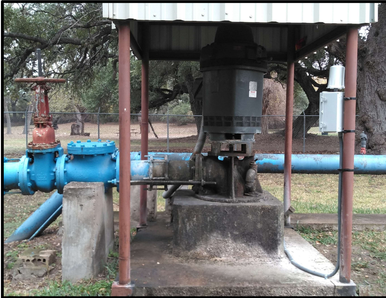
Fort Clark MUD Production Well
