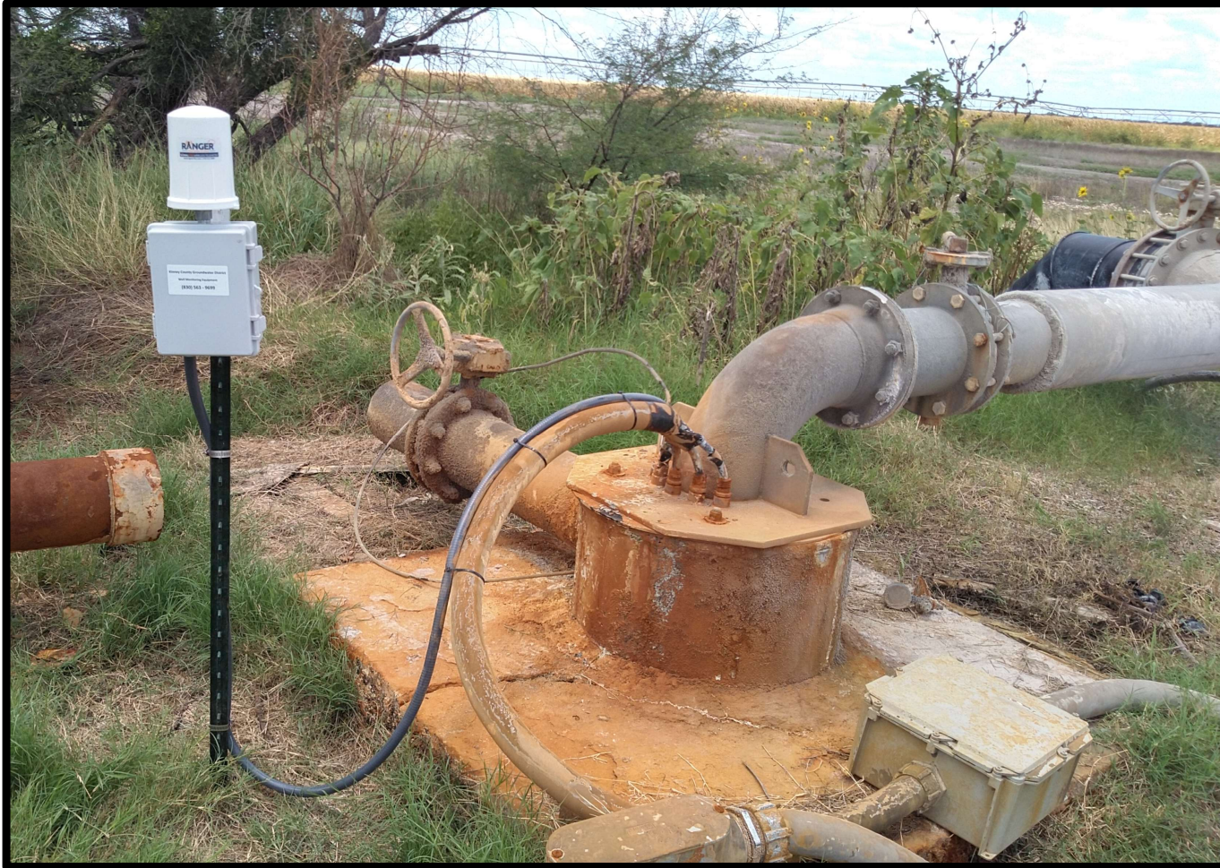
Permitted Well – Signal Fire Telemetry / Water Level
